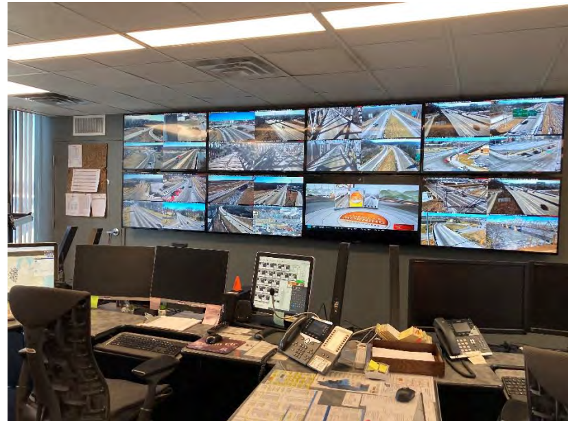
Figure 111: IDOT District 4 Communications Center in Downtown Peoria
