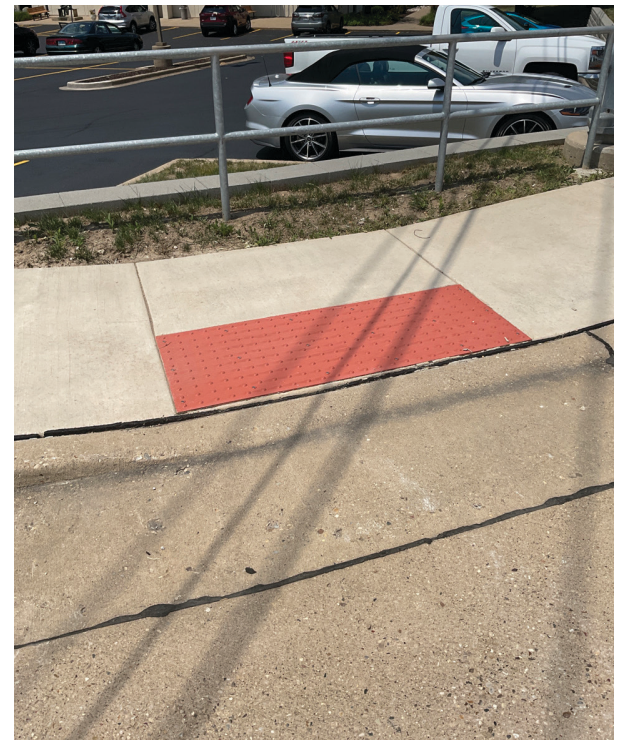
Fig. 1.22 (above) Accessible ramp with warning pad located outside Alpha Park Library on Airport Road. Map 1.4 (left) Tri-County staff inventoried sidewalk conditions in Summer 2023.
